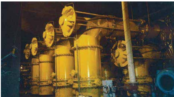
Cooling water pipes
