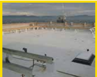
Old leaking roof.
