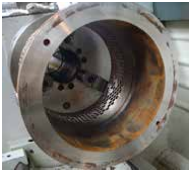
Corroded valve basket
