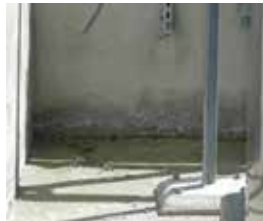
The damage had also affected the walls.
