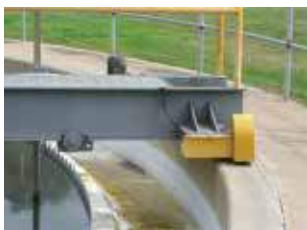
The clarifier wheel back in service.
