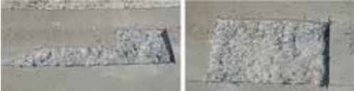
Two of the three areas of concrete that were damaged when the wheel failed.
