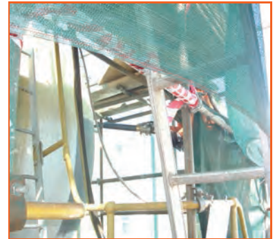
Pictured operator blasting on the end of the vessel (the grey patch is the blasted area)
